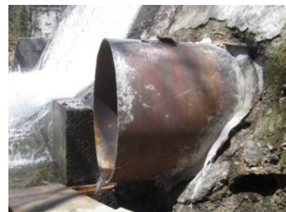
End of new sluice pipe
